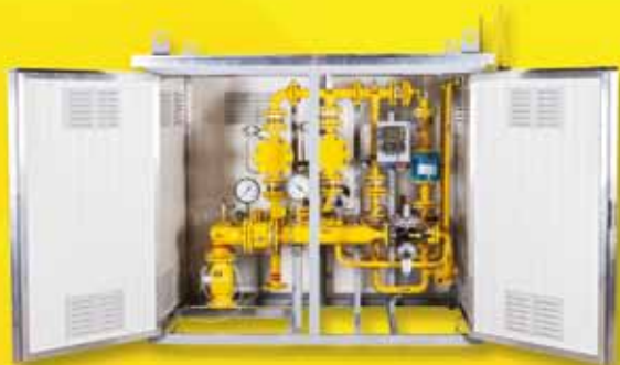
▲ Gas pressure and reducing stations (GPRM stations)
