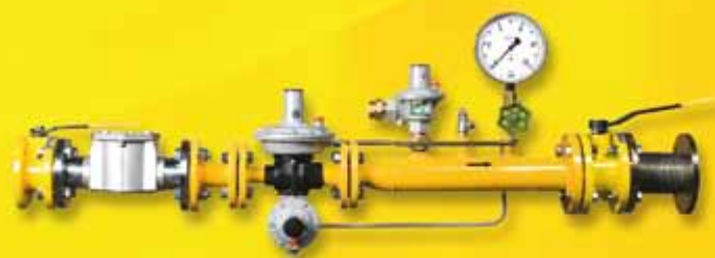
▲ Pipe fittings (gas trains)
